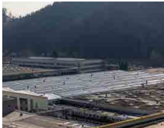
Rooftop Photovoltaics at the Gorenje d.o.o. Velenje Industrial Park
